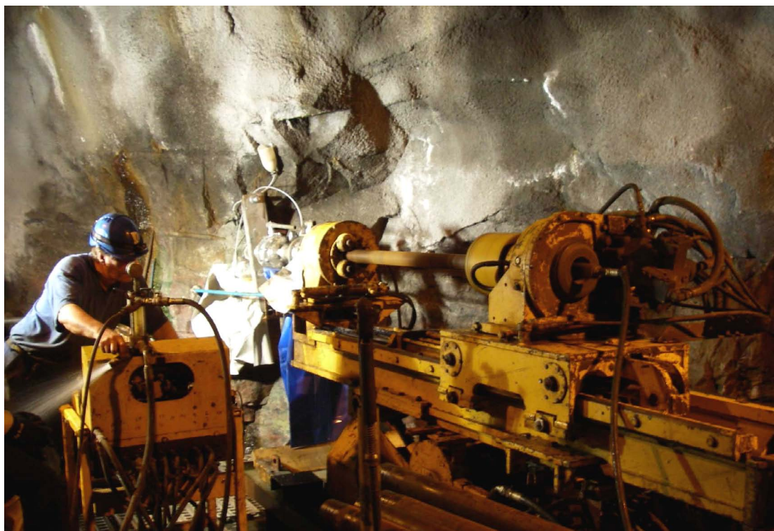
Figure 2-3. The Atlas Copco Diamec 282E drill rig at KI0016B01, it was used for the core drilling of both KI0014B01 and KI0016B01. Drillcon driller Anders Asp at the mechanical/hydraulic control unit to the left (photo: Oskar Sigurdsson).
