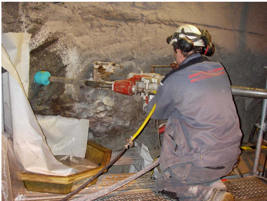
Figure 2-1. Husqvarna 406HL drill rig used for the casing drilling, driller is Mikael Gustafsson, Smålands Betonghålltagning AB. The power package is situated outside the picture (photo: Oskar Sigurdsson).
